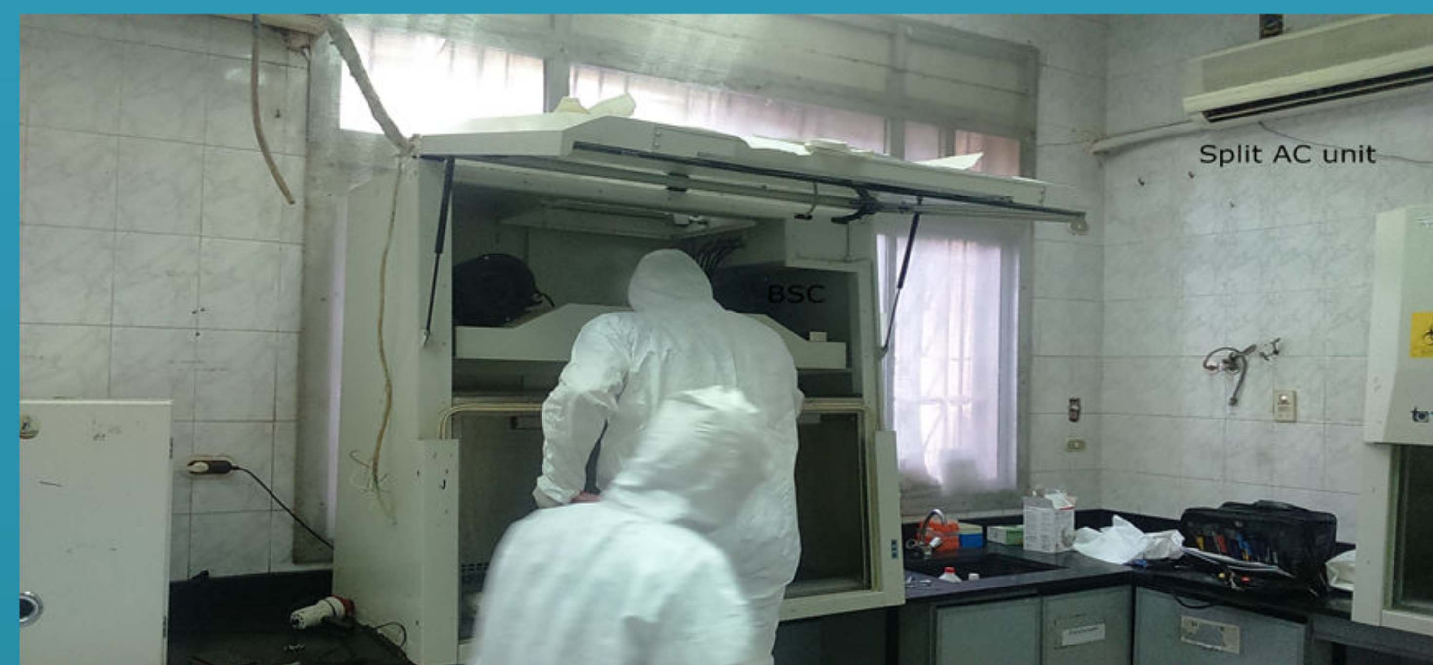
Img1: BSC positioned beside AC split unit
